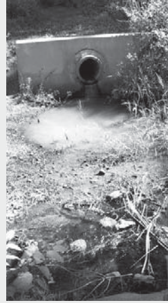
Outfall pipe along Pine Tree Brook discharging turbid water from Milton High School grounds.
